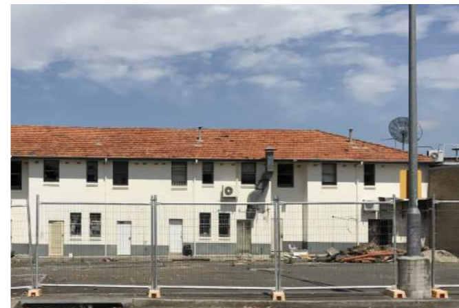
Development site on Villawood Place as seen from the Council car park at the rear (now demolished).
